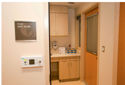
▲ View from anteroom to client's isolation room with directional air-flow negative pressure ventilation system.
