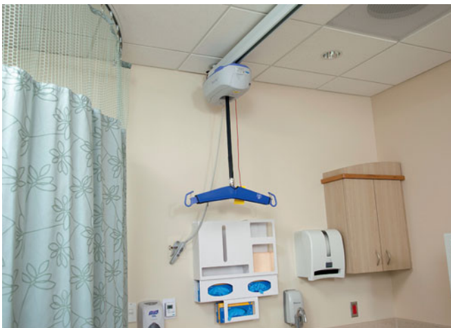
▲ Ceiling mounted lift device for client transfer.
